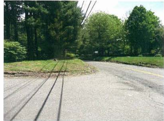
Erosion damage, longitudinal pavement cracking, and limited intersection sight distances looking east from Goodspeed Avenue
