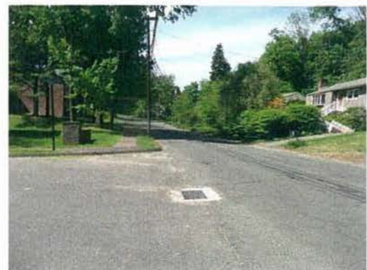
Recently installed catch basin at low point of Allen Avenue at Stoddard Drive
