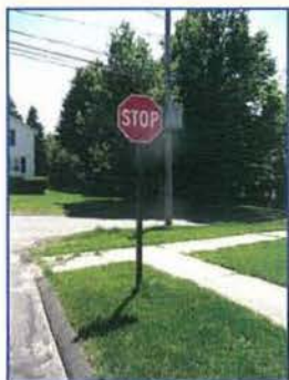
RECONSTRUCT SIDEWALKS AND RAMPS TO CONFORM TO ADA STANDARDS ALLEN AVE. AT WESTFORT DR.
