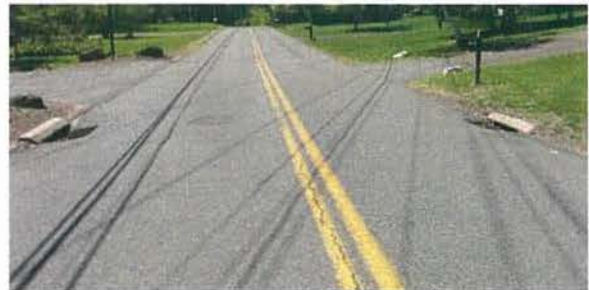
Longitudinal cracking down center line with depressed catch basins and reduced curb reveal on Allen Avenue
