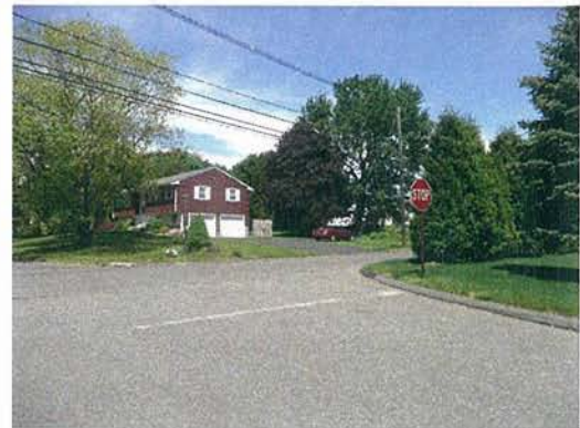
Evergreen shrub row on Allen Avenue limits intersection sight distance on Old Gate Lane looking east
