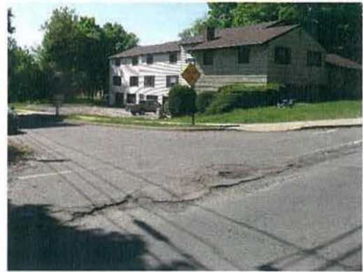
Joint cracking at Allen Court Intersection
