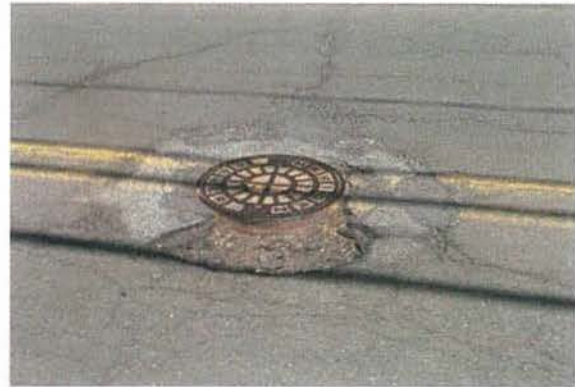
Severe pothole on Allen Avenue
