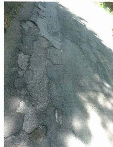
Poor pavement condition on Allen Avenue
