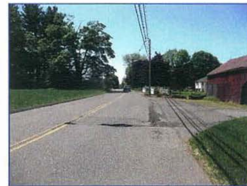
ROADWAY RECONSTRUCTION FOR PAVEMENT REHABILITATION ALLEN AVE. BETWEEN WESTFORT DR. & EDGEMARK ACRES
