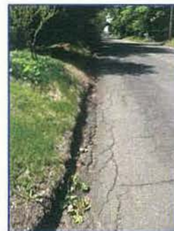
RECONSTRUCT ROADWAY DUE TO EDGE OF ROAD EROSION ALLEN AVE. WEST OF KRYVEL RD.
