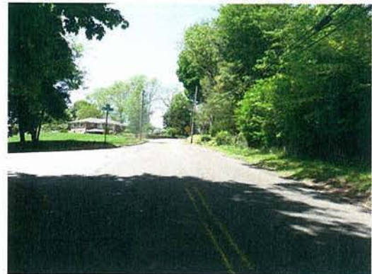
Reverse superelevation around curve north of Pasture Lane
