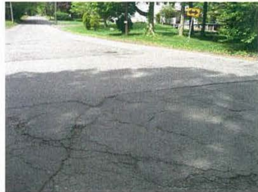
Pavement cracking at Allen Avenue and Coe Avenue intersection
