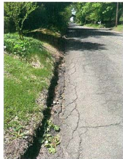
Erosion and pavement cracking along Allen Avenue
