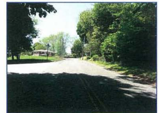
RECONSTRUCT ROADWAY TO ELIMINATE IMPROPER SUPERELEVATION ALLEN AVE. AT PASTURE LANE LOOKING WEST
