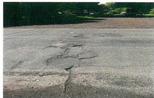
Severe pavement cracking and potholes on Johnson Avenue at Fairfax Avenue intersection
