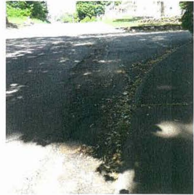
Poor pavement condition at Johnson Heights Intersection
