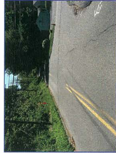
RECONSTRUCT ROADWAY TO FLATTEN VERTICAL PROFILE JOHNSON AVE. AT FINCH AVE. LOOKING EAST
