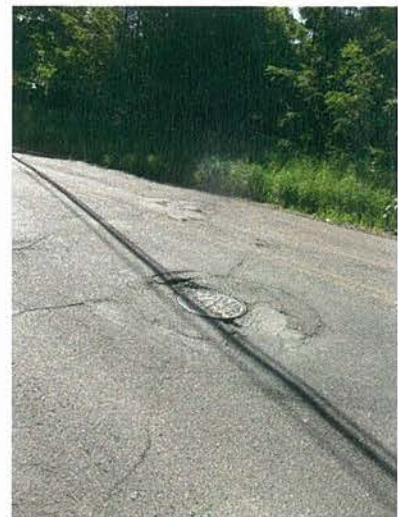
Poor pavement condition around manholes on Johnson Avenue
