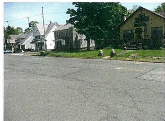
Pavement patches, cracking, faded pavement markings and two stop bars present on Johnson Avenue at West Main Street Intersection
