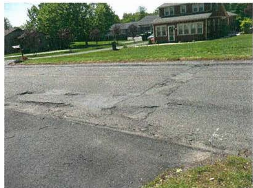
Poor pavement condition on Johnson Avenue
