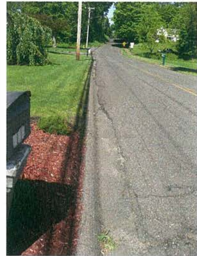
Erosion of pavement layers along Johnson Avenue
