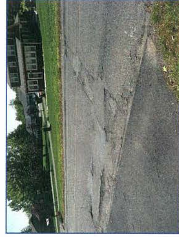
RECONSTRUCT ROADWAY FOR PAVEMENT REHABILITATION JOHNSON AVE. BETWEEN SPERRY LN. AND EATON AVE.
