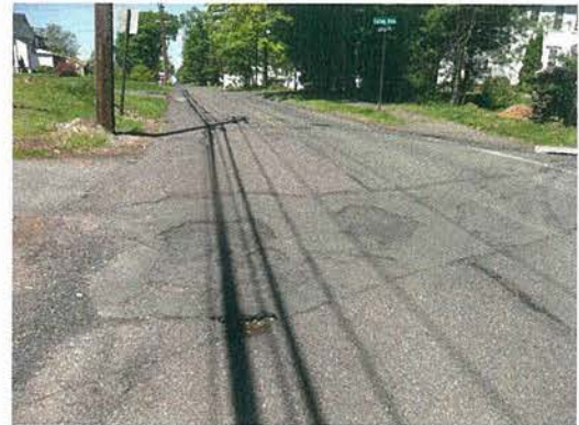
Poor pavement condition at the Eaton Avenue intersection
