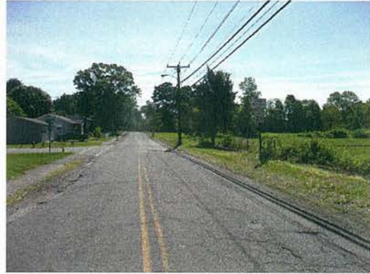
Fatigue cracking at the intersection of Johnson Avenue and Smithfield Avenue
