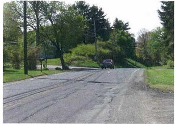
Preston Avenue southbound approach to Clearfield Drive intersection shows extensive
