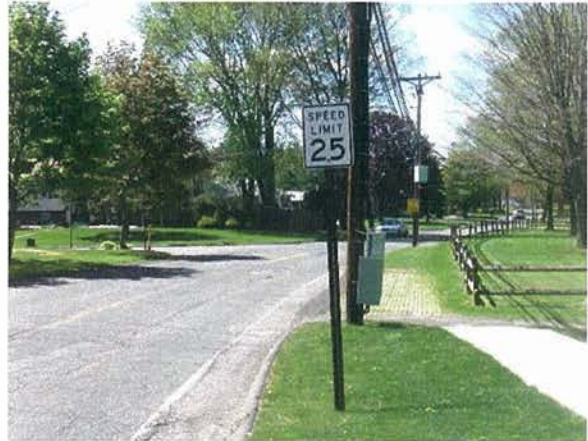
Sidewalk gap on westbound Baldwin Avenue approach to intersection with Higby Drive
