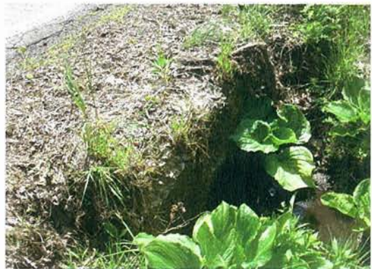
Top: Drainage basin, damaged highway sign, fatigued pavement, and incomplete sidewalk Bottom: Unprotected outlet across the street from the catch basin
