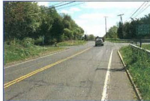
PRUNE VEGETATION TO IMPROVE SIGHT DISTANCE JOHNSON AVE. AT POLICE ACADEMY DR. LOOKING SOUTH
