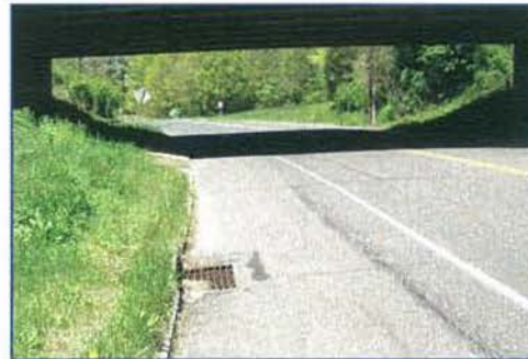
SUBSTANDARD VERTICAL CLEARANCE UNDER I-91 BALDWIN AVENUE LOOKING WEST UNDER I-91
