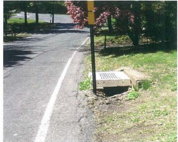
Protruding drainage inlet on southbound Preston Avenue before intersection with East Main Street
