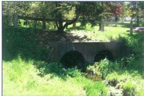
UPGRADE ROADSIDE PROTECTION AT CULVERT JOHNSON AVE. AT FAIRFAX AVE. LOOKING EAST
