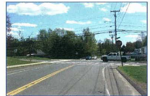
PRUNE VEGETATION TO IMPROVE SIGHT DISTANCE BEE ST. AT BALDWIN AVE. LOOKING SOUTH
