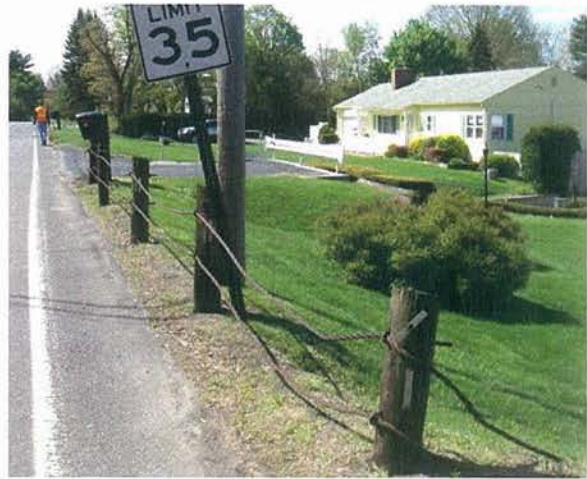
Inadequate barrier on southbound lane of Preston Avenue
