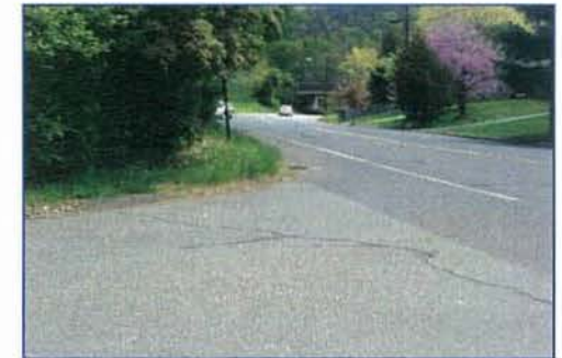
MILL AND OVERLAY EXISTING PAVEMENT BALDWIN AVE. AT PRESTON DR. LOOKING WEST
