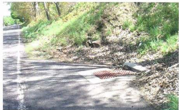
Drainage basin on northbound (cut) side of Preston Avenue north of Patton Drive
