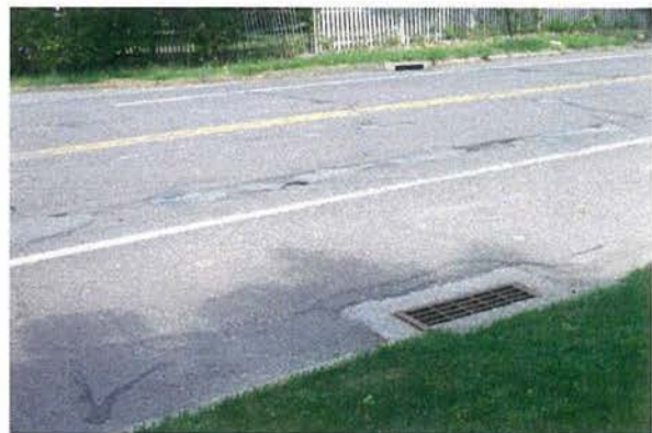
Drainage and pavement condition on Baldwin Avenue east of Preston Drive
