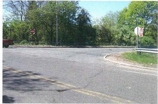
Outdated cable guide railing on Route 66 off-ramp
