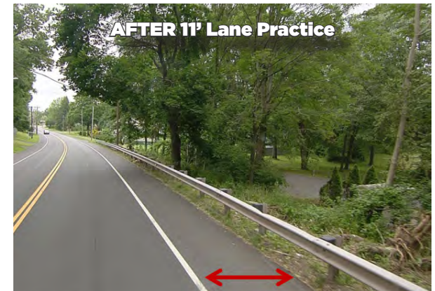
An example of a shoulder widening as a result of the VIP Paving Program (Image credit: CTDOT)
