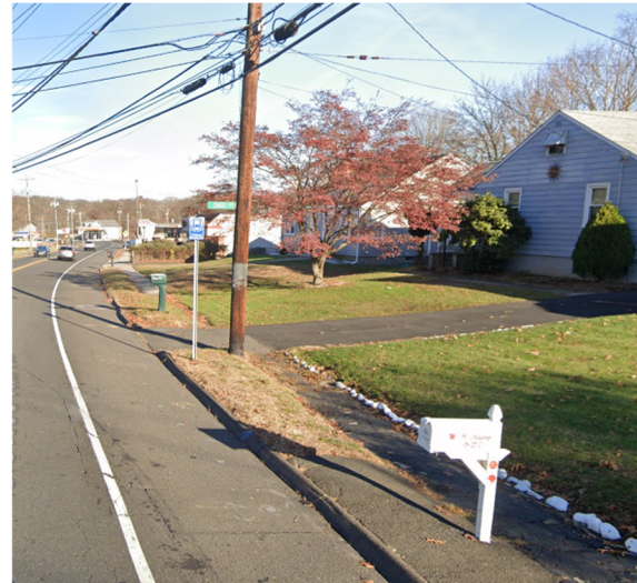
Poor quality sidewalk along the south side of Jones Hill Road across from Edith E. Mackrille Elementary School (Source: Google Maps)
