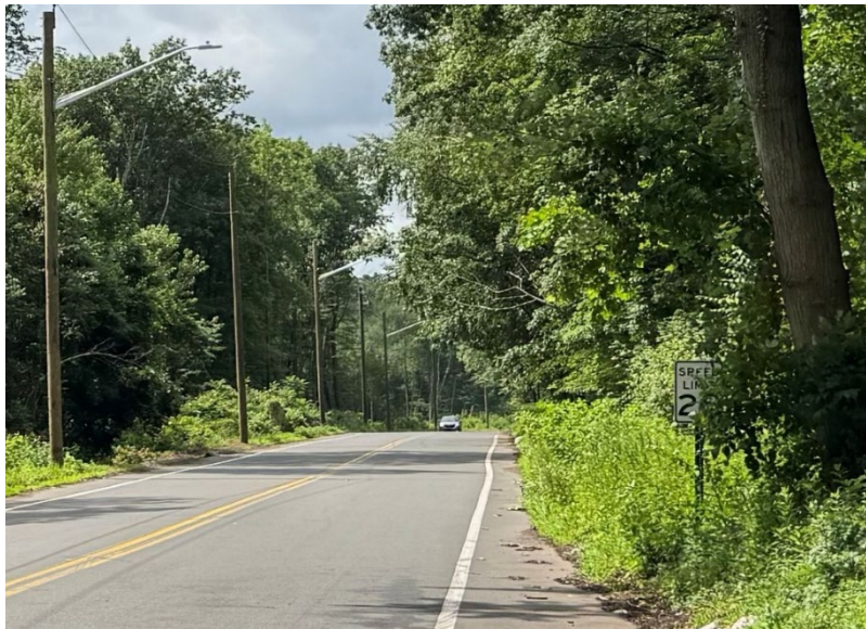
Figure 8 Obscured Speed Limit Sign on Valley Service Road
