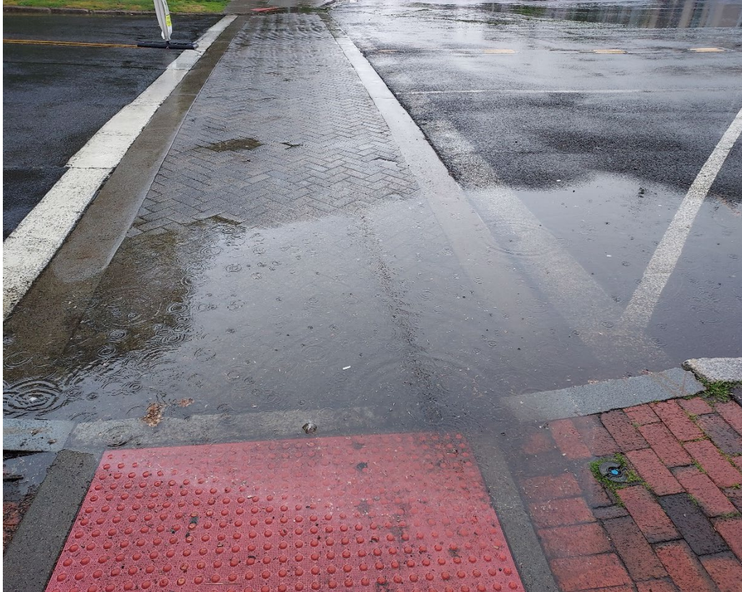
Figure 9 Flooded Curb Ramp – Whitfield Street at Boston Street
