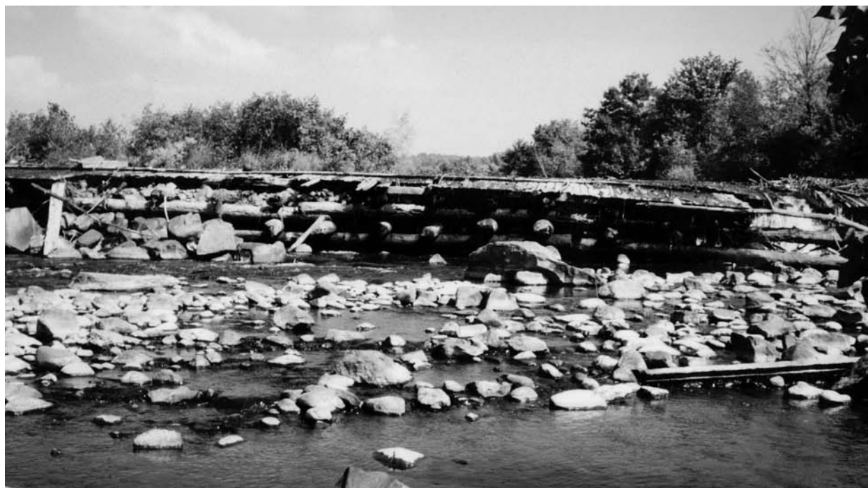
Anaconda Dam on the Naugatuck River in Connecticut. Photo: Laura Wildman, Milone and Macbroom.
